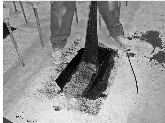
Figure X – Adhesive failure (fail)
