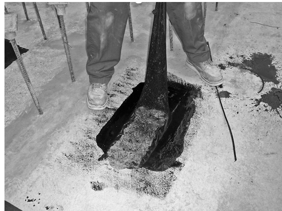
Figure X – Adhesive failure (fail)
